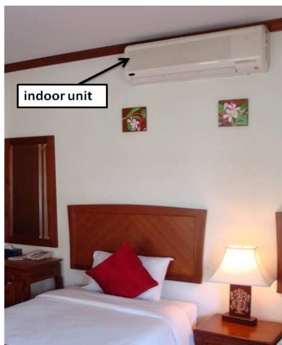
(Air conditioner – indoor unit)
