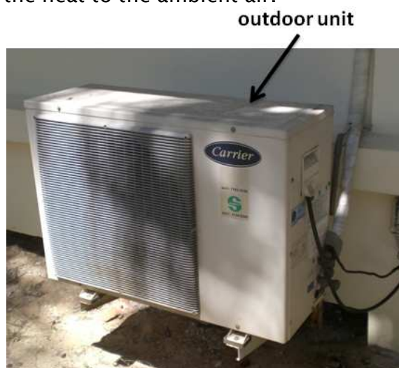
(Air conditioner – outdoor unit)
